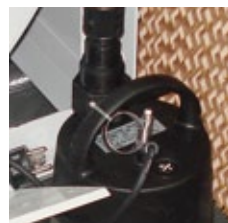
GRUNDFOS WATER PUMP WITH FLOW REGULATION AND CONTINUOUS DRAINAGE SYSTEM TO AVOID MINERAL SALT CONCENTRATION.
