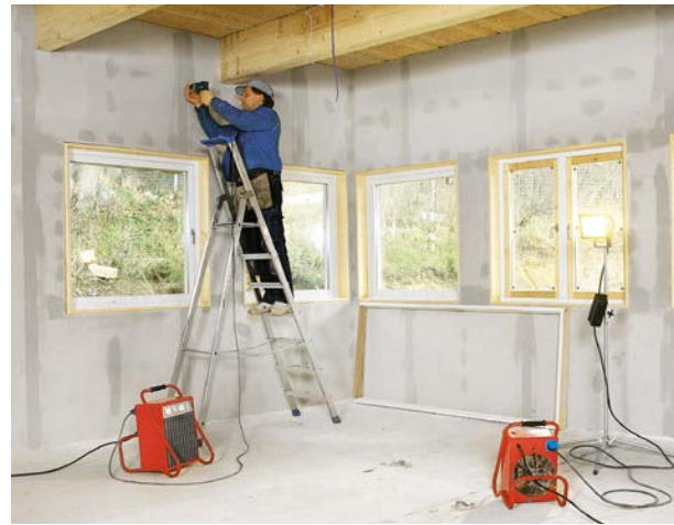
Tiger 3-9 kW (400V3N~) has a 230V outlet at the rear for easy connection of e.g. lighting or a charger for cordless tools. Practical for building sites!
