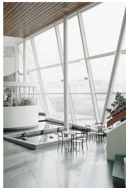
Thermoplus is used for cold draught protection. The radiant heat moulding is very discreet as it is positioned high up along a beam.
