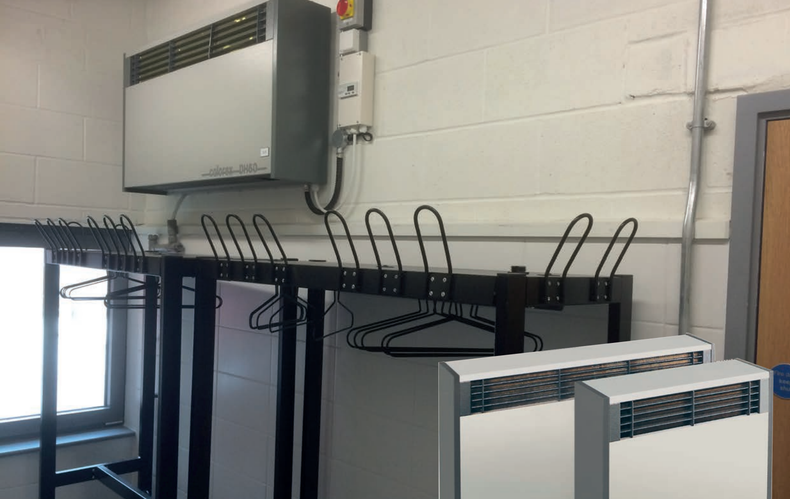
A Calorex DH60 installed in the drying room of Orpington fire station
